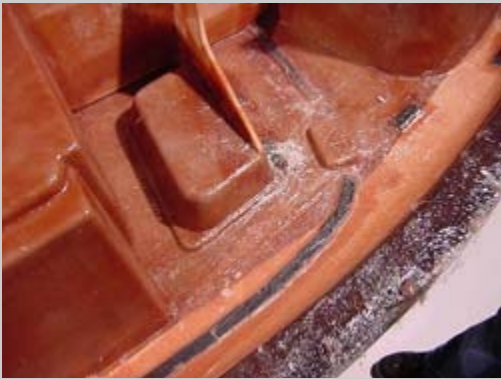
Glassed in strip of HDPE (in black) where the windshield will be installed
