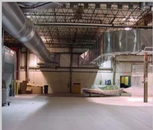
Gelcoat spray booth ventilation system
